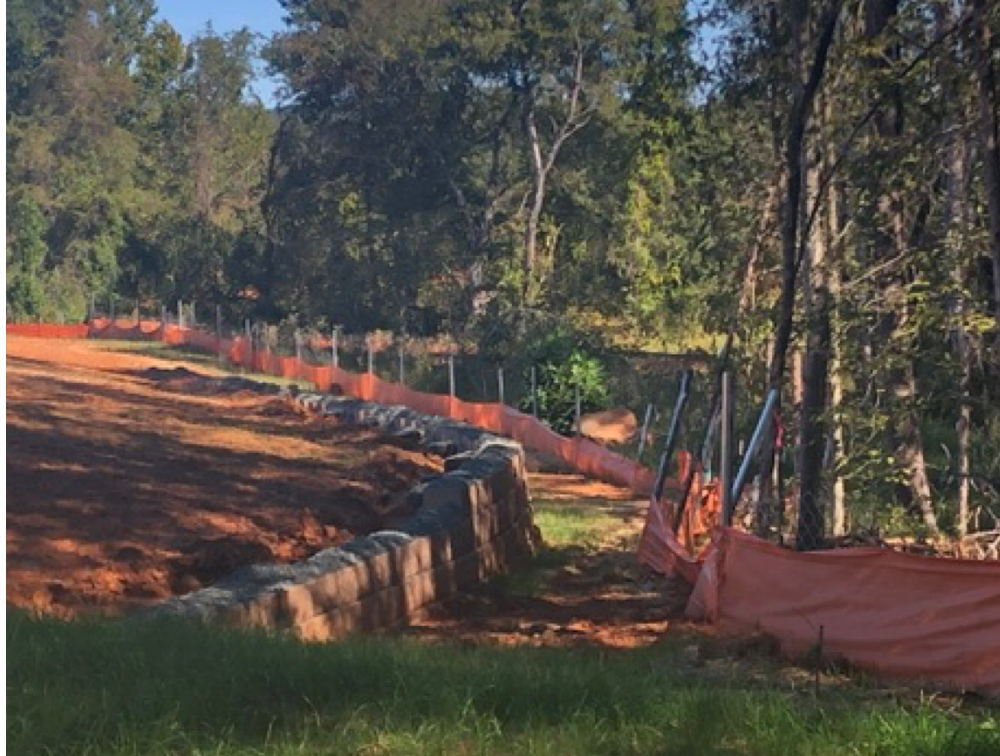
Figure 2. Photograph of over-clearing at Glenbrook at Parkside, extending into the designated stream buffer (stream is located behind trees at right of photo). No trees in this area have been replaced. Photo taken September 26, 2021.
