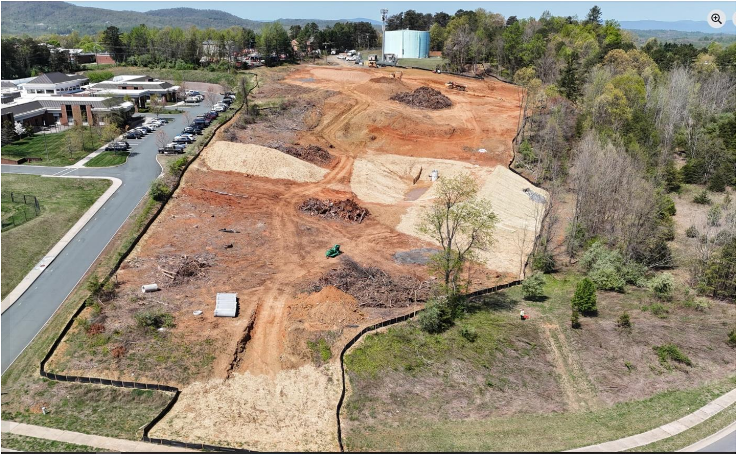
Image (from ACSA Facebook page dated May 2025): Looking west at ACSA Property under construction
