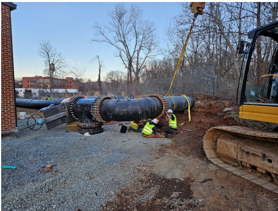
Bypass system pipes.
