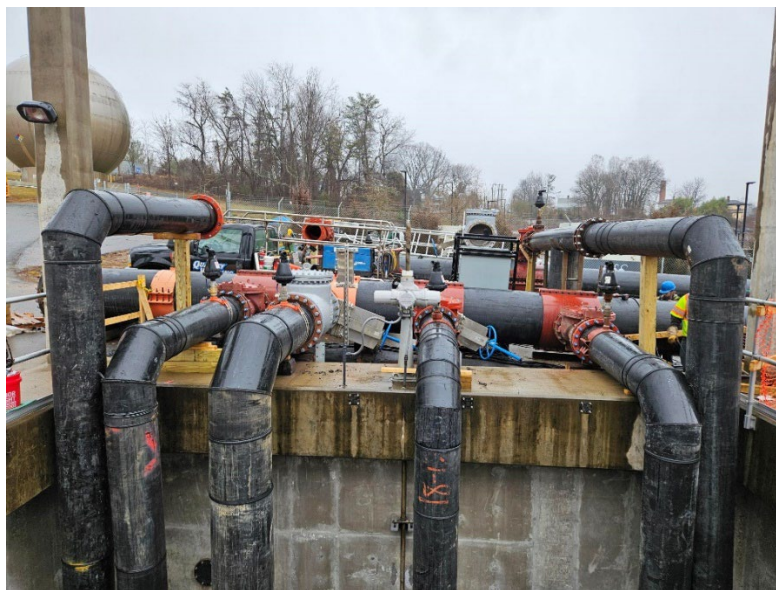
55 million gallons per day bypass pumping system
