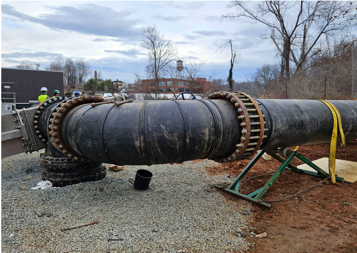
55 million gallons per day pumping bypass system
