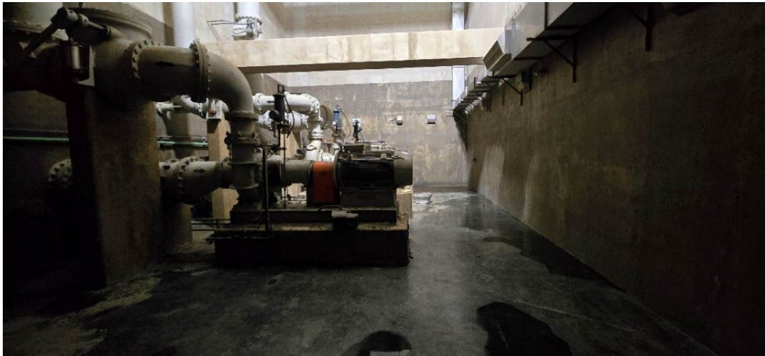
Cleaned pump room.
